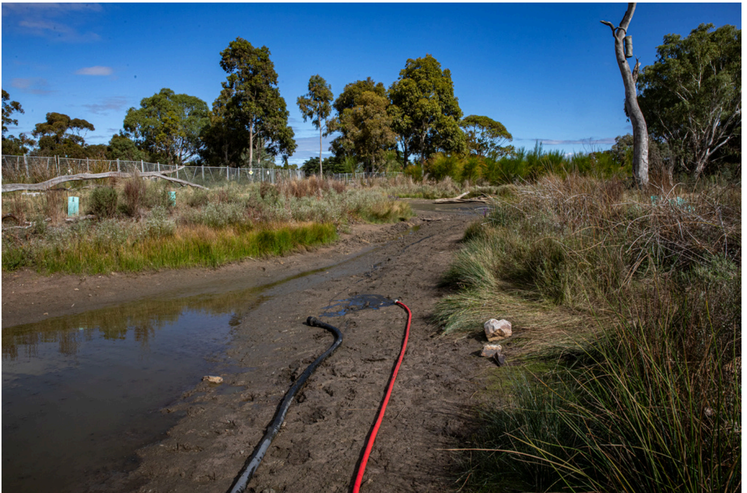
YWNA teams were actively pumping out water to facilitate the drying process
